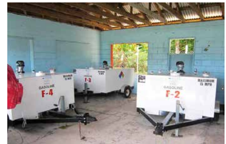
Transportable fuel tanks.
